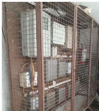
Electrical Panel in Safety Cabinet
