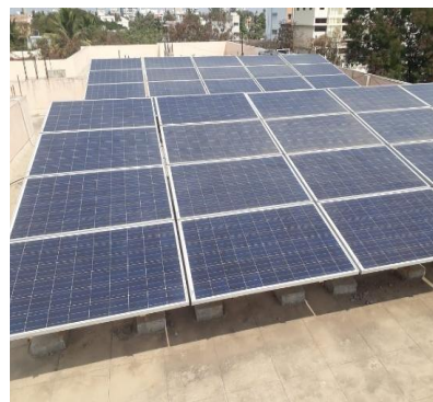
Solar Electricity Generation System
