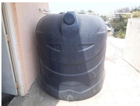
2000 Liters Drinking Water Storage Tank
