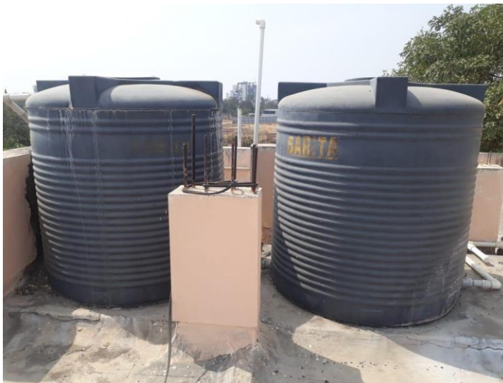
Non-drinking Water Storage Tank (each 2000 liter capacity)
