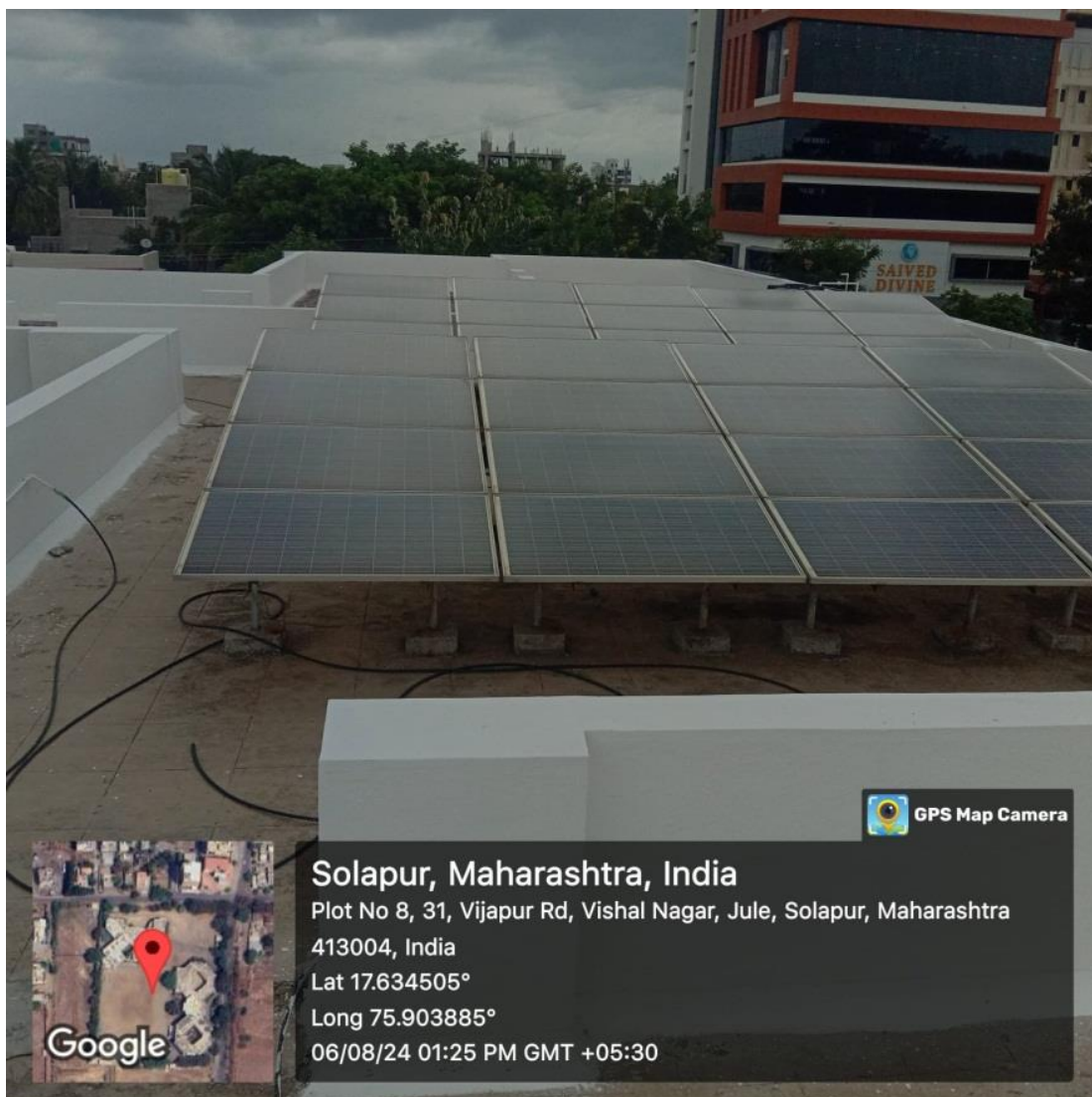
a) Use of Solar ensrgy
