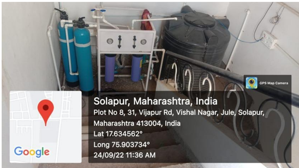
RO Water facility
