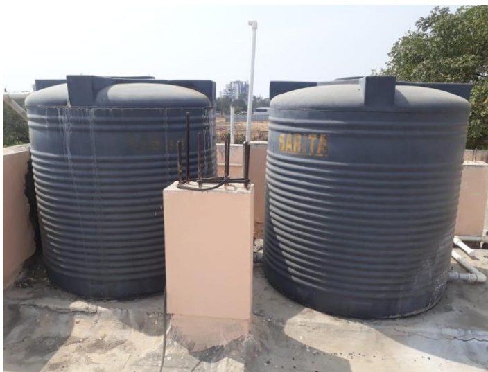
Non-drinking Water Storage Tank (each 2000 liter capacity)
