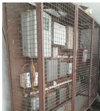
Electrical Panel in Safety Cabinet
