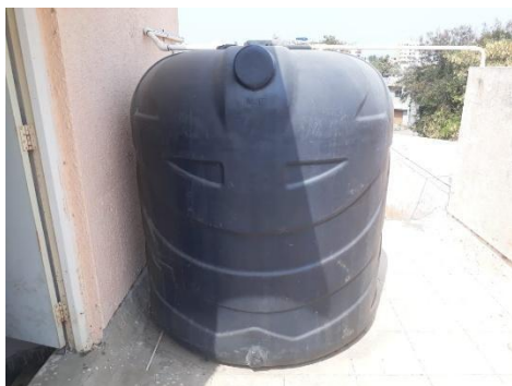
2000 Liters Drinking Water Storage Tank
