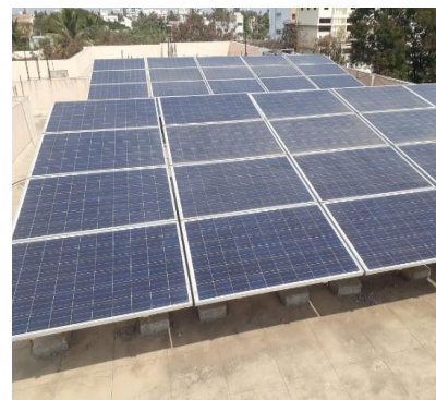
Solar Electricity Generation System
